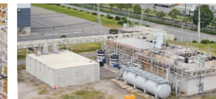
Ako Plant wastewater treatment facility
