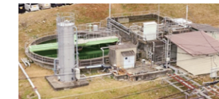
Sakoshi Plant wastewater treatment facility
